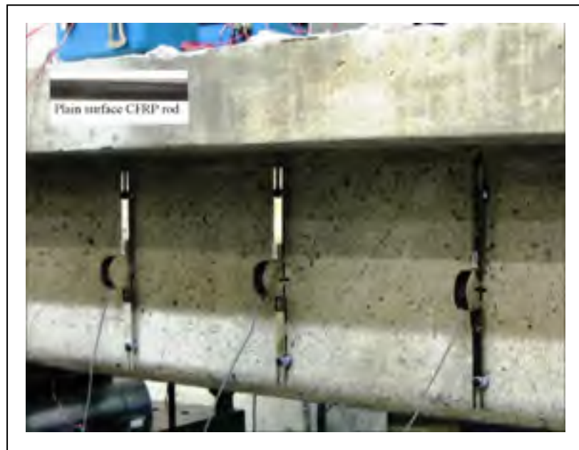
Figure 7.5 Parallel diagonal shear cracks, specimen S1-9d-260p.
