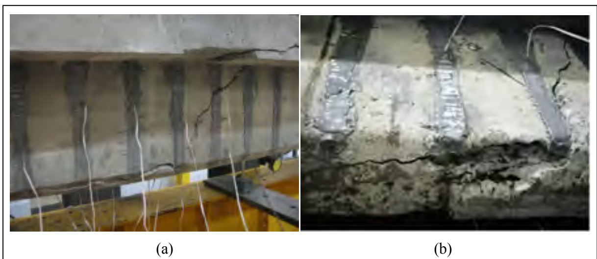
Figure 4.4 Common failure mode in beams strengthened with NSM method: a) Cracking pattern and b) detachment of concrete cover.
