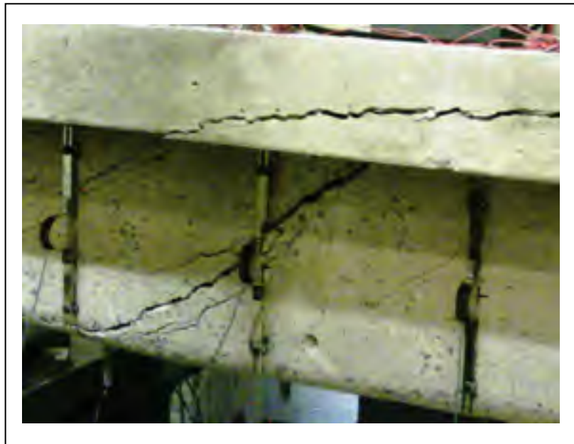
Figure 7.7 Failure mode of specimen S1-9d260p.
