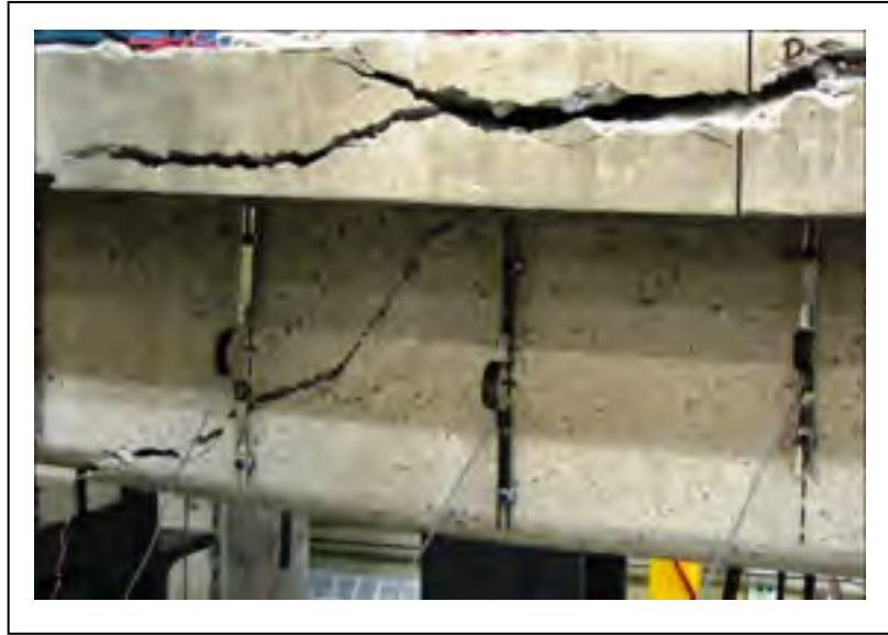
Figure 7.6 Failure mode of specimen S1-9d260s.
