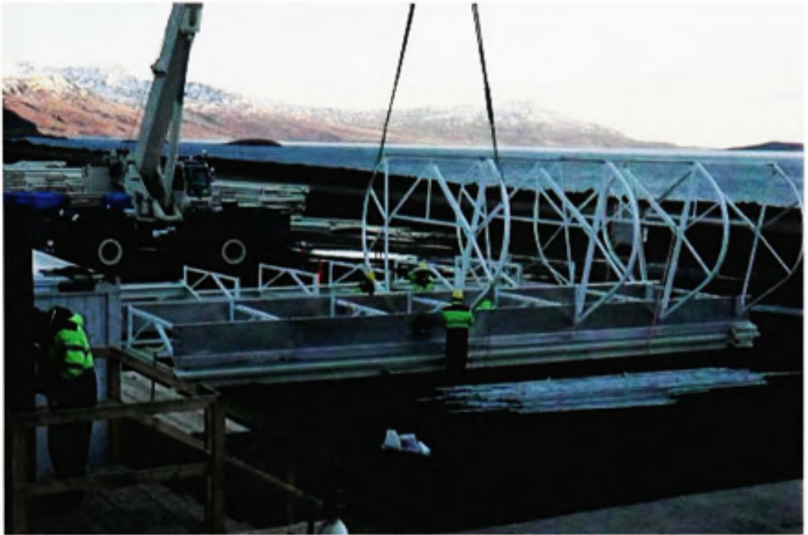
Air-Therm ventilator module being assembled on the ground: due to barcode system module utilizing this system were assembled faster and utilizing less labour
