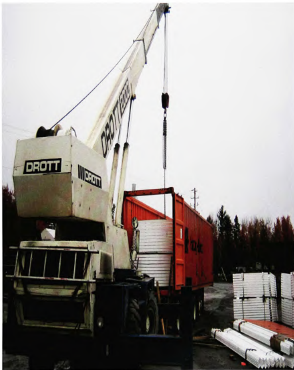
Frame components post fabrication at Air-Therm works scanned and approved being loaded for transport to jobsite
