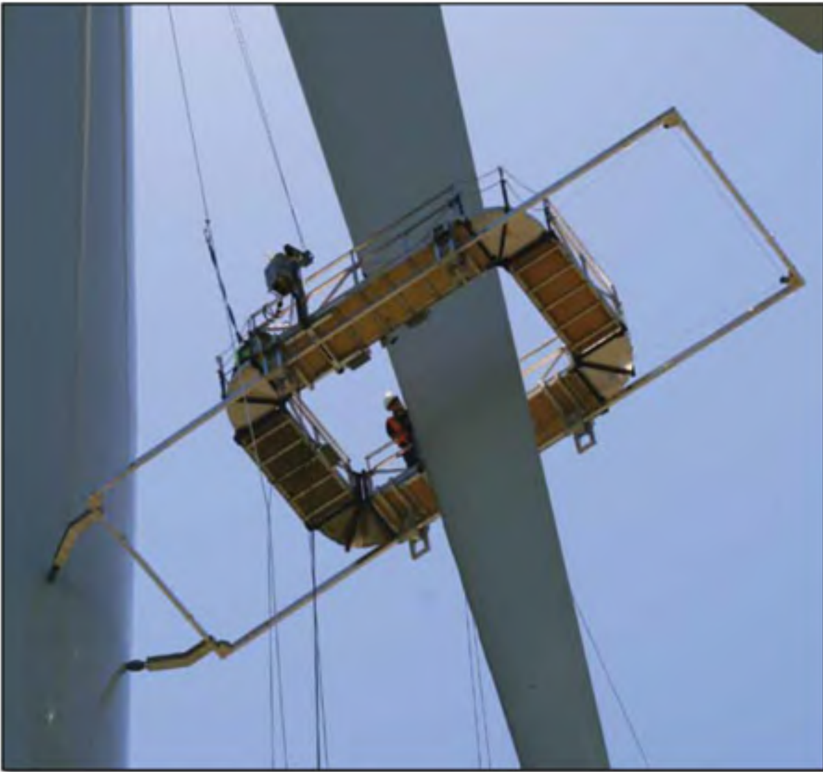
Figure 3.25 : Suspended access equipment for Wind Turbine ( www.spiderstaging.com )
