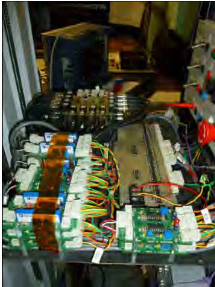
Figure-A II-5 The measurement probes, sensors protections, and IGBT firing drivers with their protections
