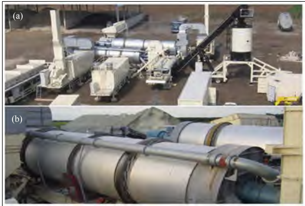
Figure 1.11 Example of the mobile parallel drum plant of AAPPIA Grands Travaux a) overall view & b) closer view of the two parallel drum dryers (the first one for virgin aggregates, the second one for recycled aggregate) Taken from Olard et al. (2008)
