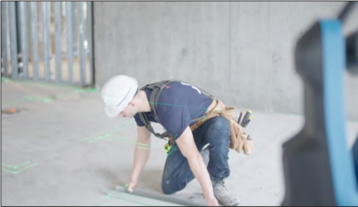
Figure 5.5 Laser projection of interior division plane on a concrete slab by FramR of Mechasys
