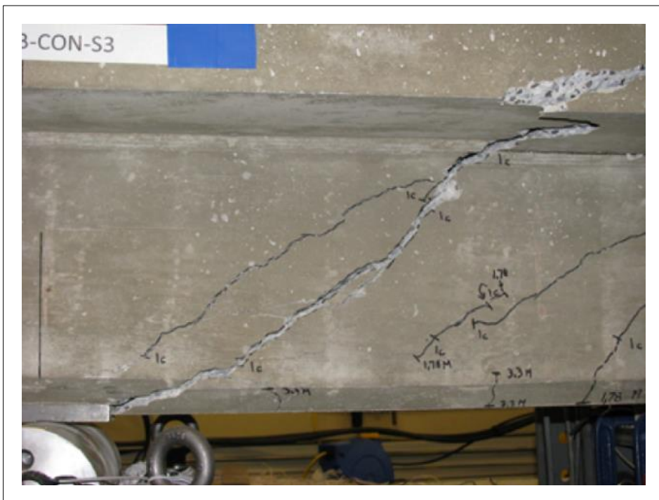
Figure 1.1 Shear failure of an RC beam Taken from El-Saikaly and Chaallal (2015-b)
