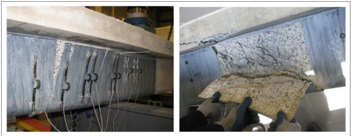
Figure 1.6 FRP debonding failure in an EB-FRP strengthened RC beam Taken from El-Saikaly and Chaallal (2015-b)
