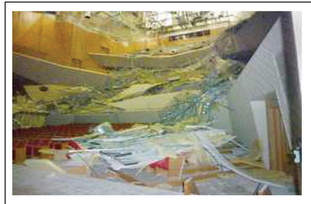
Figure 1.3 Collapsed ceiling of the Kawasaki concert hall after the 2011 Tōhoku earthquake Taken from Wang and Dai (2014, p. 1)
