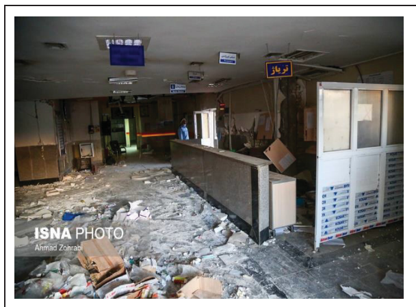
Figure 1.4 Imam Khomeini Hospital after the 2017 Ezgeleh (Kermanshah, Iran) earthquake Taken from Zohrabi, ISNA News Agency (2017)
