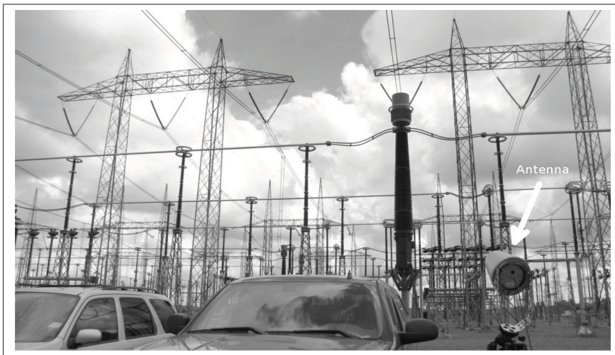
Figure 2.3 Typical HV equipment in the 735 kV substation
