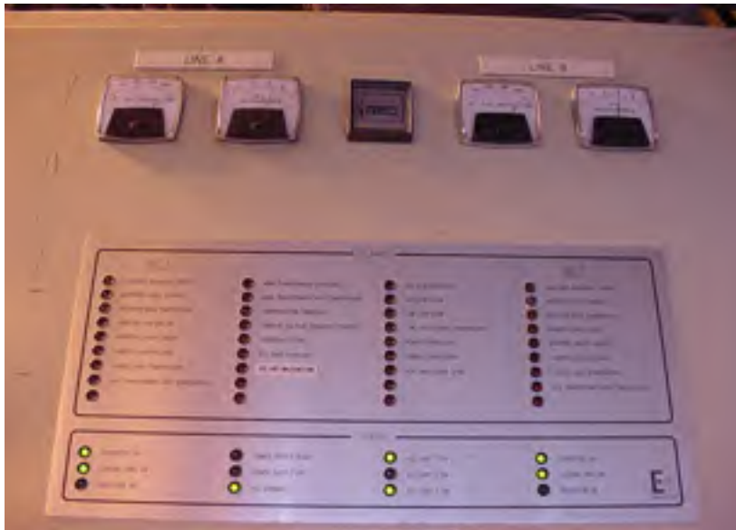
Figure 6.7 Door-mounted alarm annunciator and analog meters
