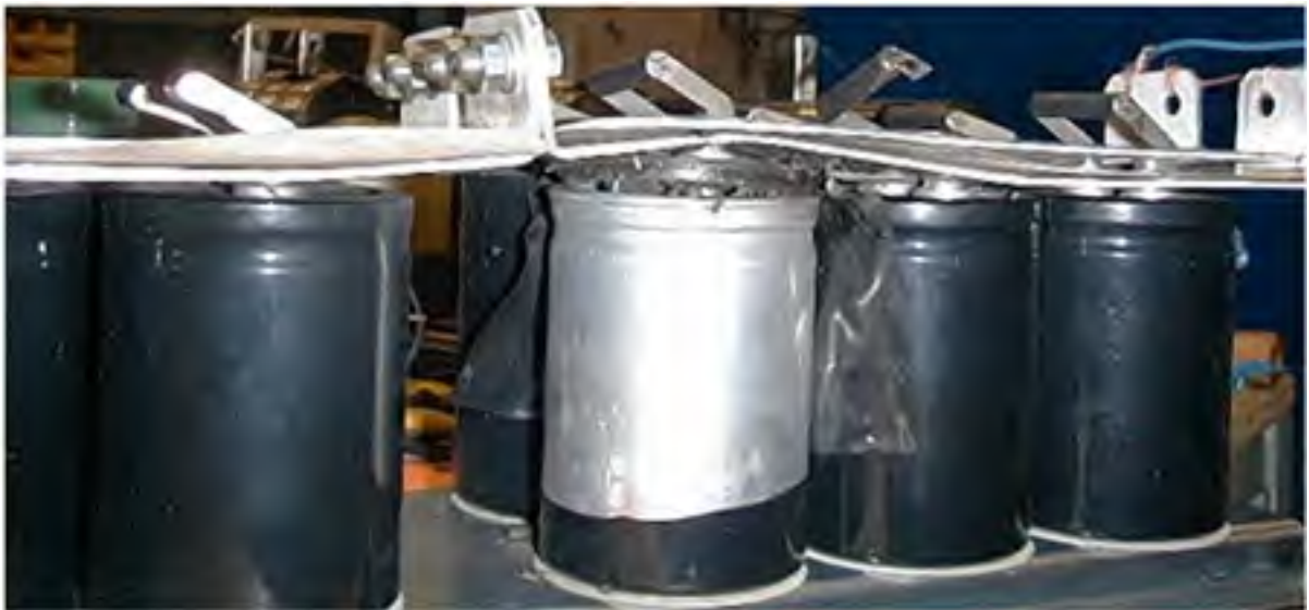
Figure 3.24 Damage to a capacitor bank from imbalanced series connection
