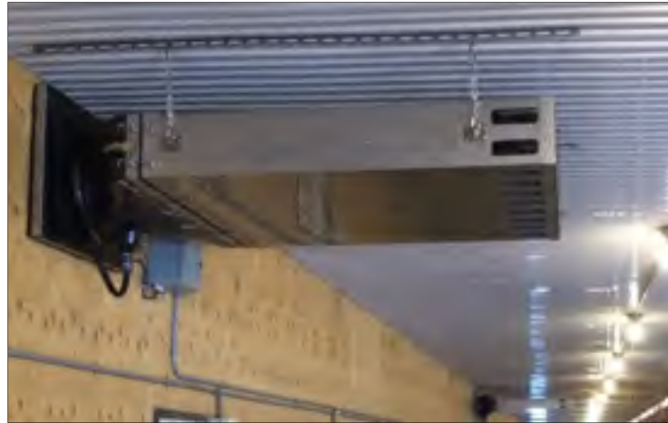
Figure 2.3 Counter-flow air-to-air HX unit installed in a broiler house
