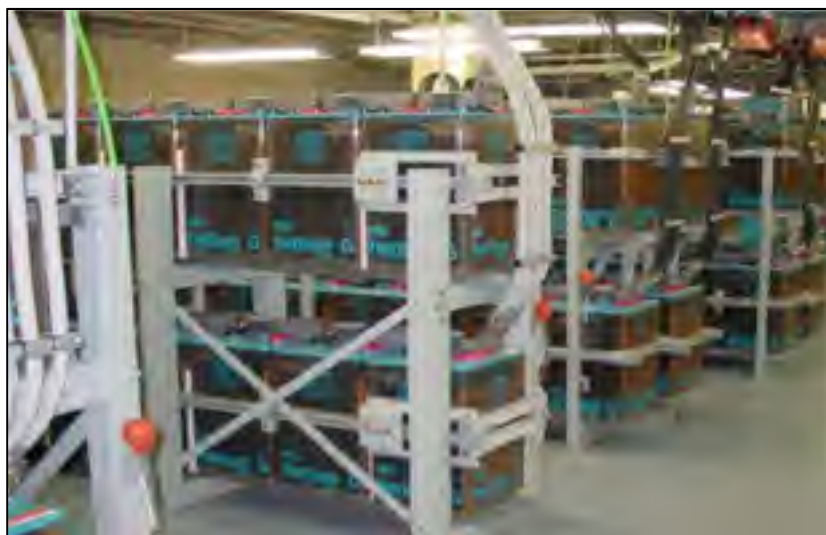
Figure 6-13 Layout of Battery Cells Room Taken from IEEE – Lead Acid Battery Fundamentals Presentation
