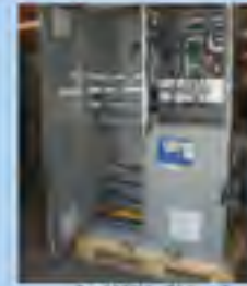
2 x 12376w-734 with battery cabinet
