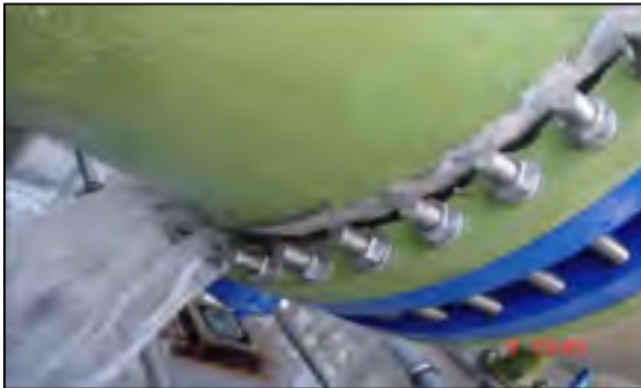
Figure 1-26 Crack at hub neck of the flange (Dynaflow 2011)
