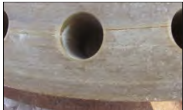
Figure 1-25 Crack in the flange face between the bolts and inside the bolt hole (Dynaflow 2011)
