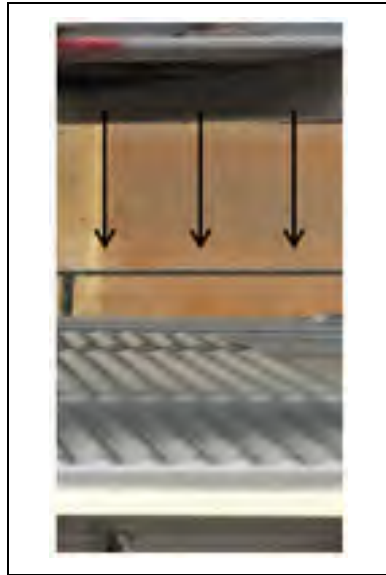
Figure 4-4 The SPF part under the cooling fans
