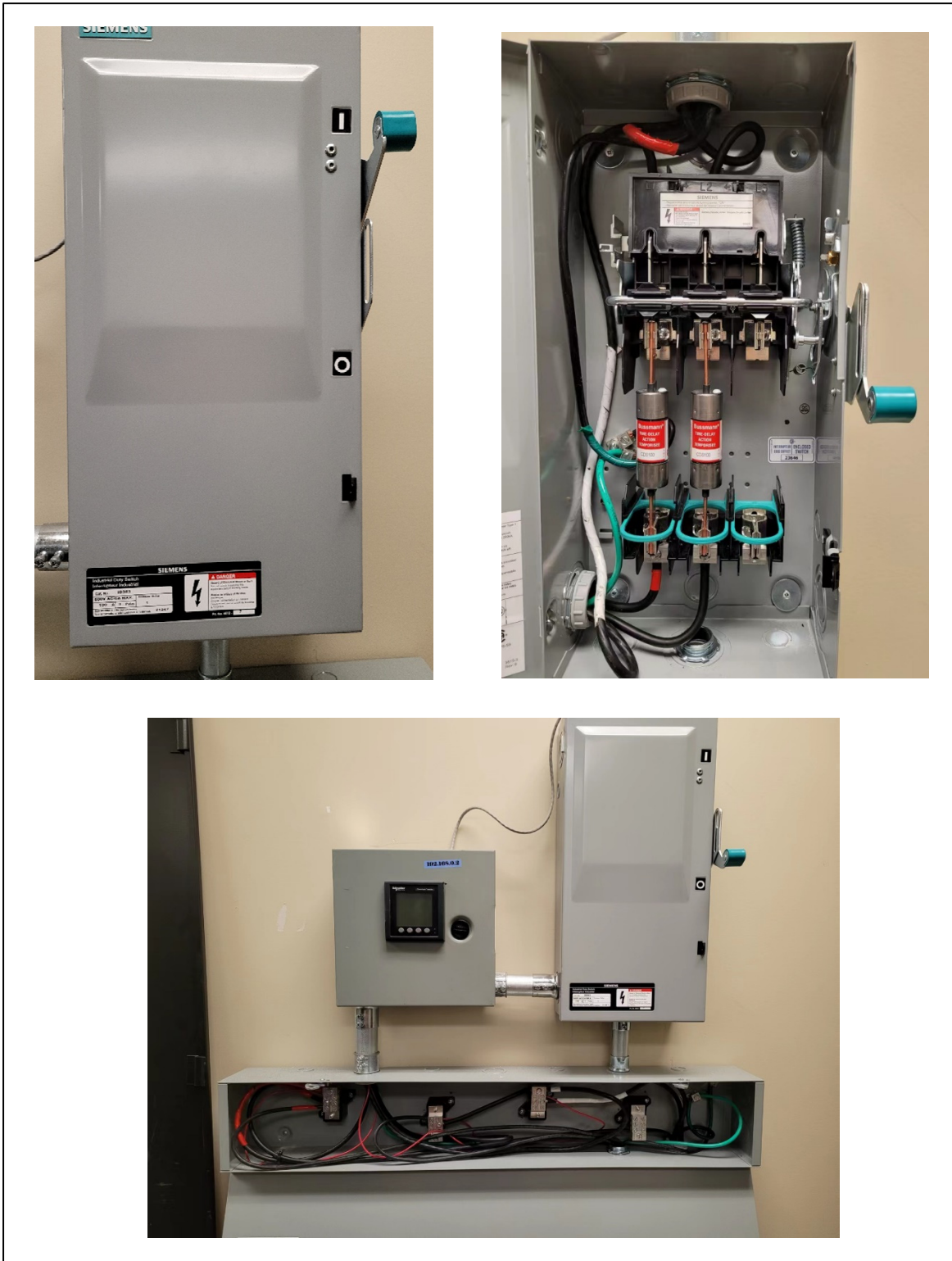
Figure 2.4 MG Gateway Cabinet
