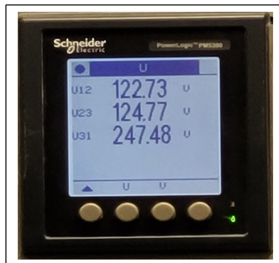
Figure 4.9 Grid Voltage Read from HMI
